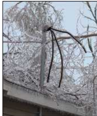
Weatherhead with lines cut by an Electrician
